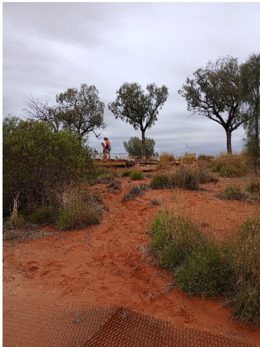
Figure 14 Construction site of Camp 2, showing footprints between sleeping platforms and access walk, 13/02/2026
