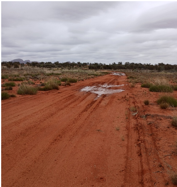
Figure 22 Access Road to Camp 2, showing water puddles and vehicle tracks, 13/02/2026
