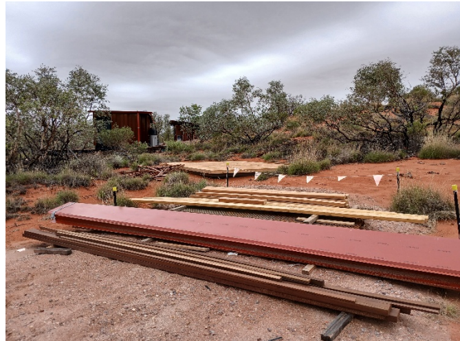
Figure 5 Construction site of Camp 1, showing piles of material, flagging fence, staff sleeping platform and Wiltjas, 13/02/2026
