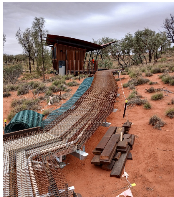
Figure 9 Elevated steel mesh walk at Camp 1, with pile of construction material on top of flagging fence, 13/02/2026
