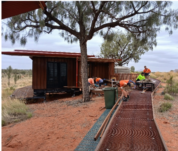
Figure 10 Construction works at Camp 2 at big Wiltja, showing metal access path and construction workers carrying in materials with a big trolley, 13/02/2026
