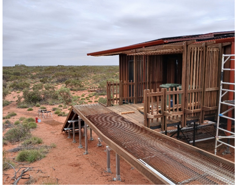
Figure 17 Construction site of Camp 3, showing “Chill Room” Wiltja and steel mesh walk to Storytelling area, 13/02/2026
