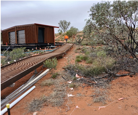
Figure 6 Construction site of Camp 1, showing big Wiltja accessible by an elevated steel mesh walk and a degraded flagging fence, 13/02/2026
